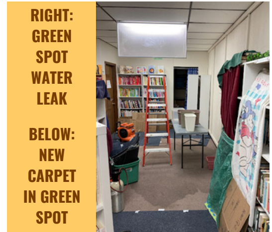
RIGHT: GREEN READ WATER LEAK
